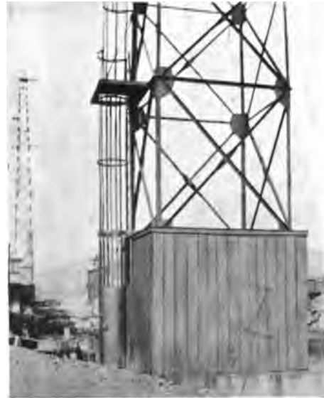
Fig. 2. Safety Cage on Ladder of High-Tension Tower.*
